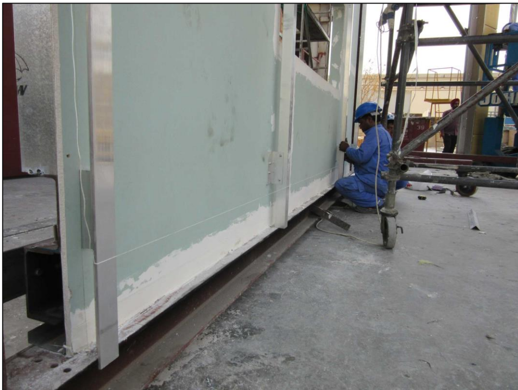
Picture 2: Aluminium brackets fixed onto the steel channels through the base wall.
