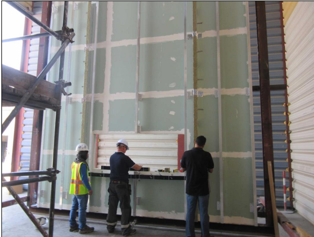
Picture 3: SIDERISE RV/RH fire barrier system being fixed onto the base wall.
