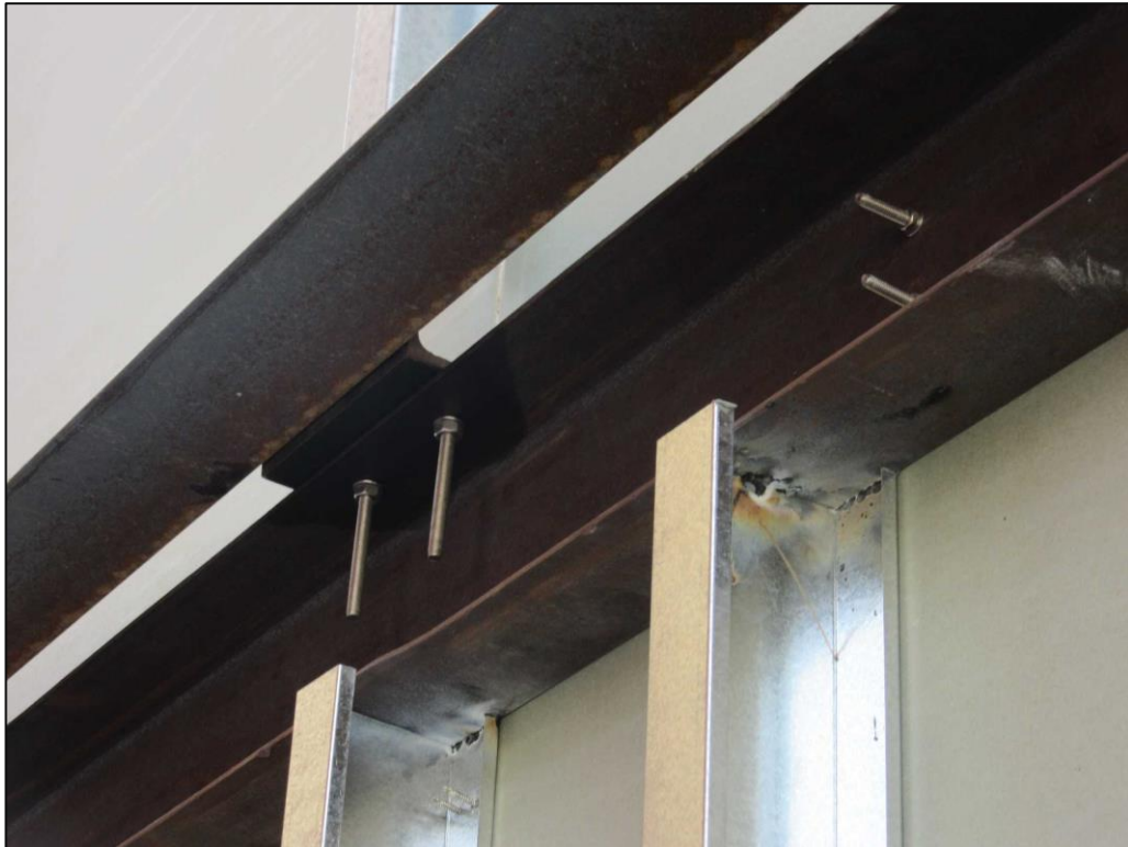
Picture 1: Steel channel system to hold the framing system of the assembly.
