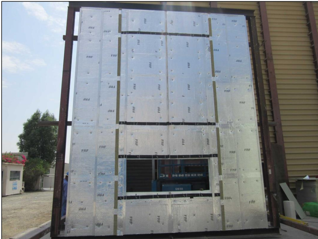
Picture 6: The specimen after the insulation and fire barrier systems were installed.
